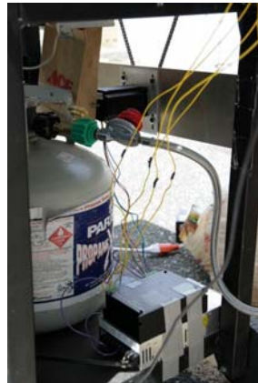
Figure 11. Gas and Flip Control Systems
